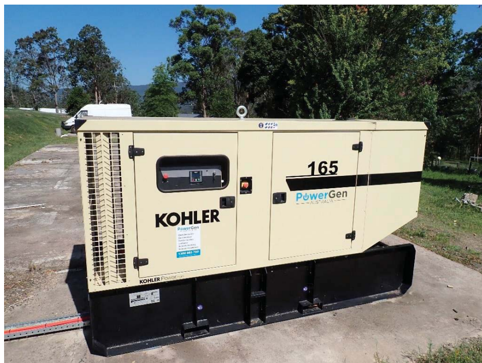
Photograph 08: Existing backup Generator
