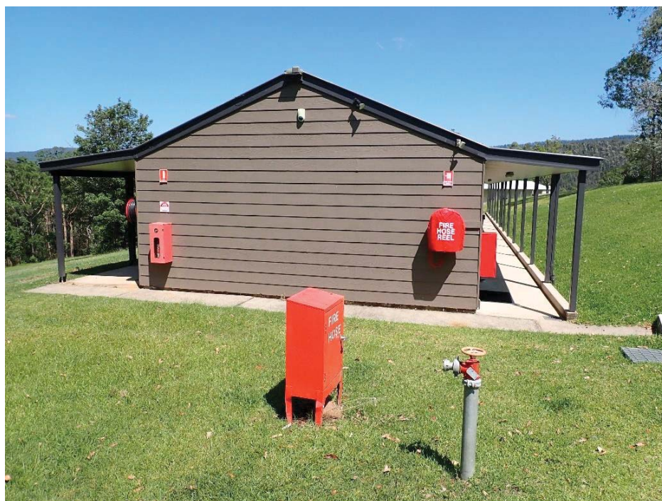
Photograph 07: Typical Fire hydrant and Hose reels
