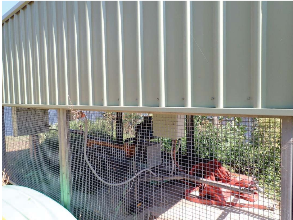
Photograph 04: Existing Pump located at Kangaroo River
