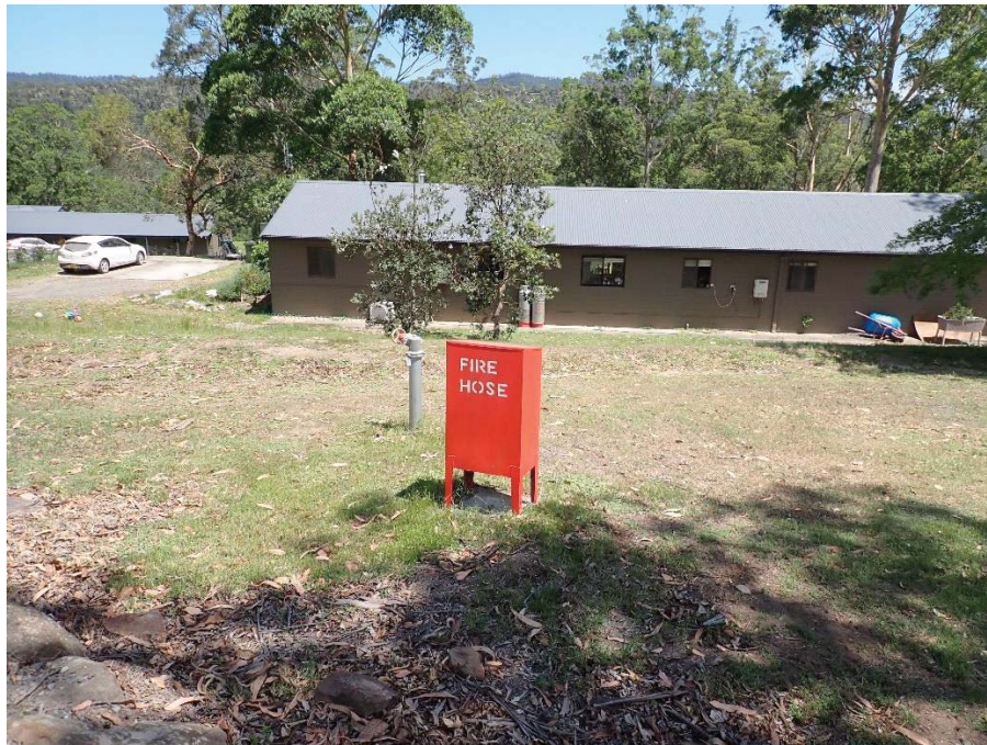
Photograph 05: Existing Pillar Hydrant and Fire Hose
